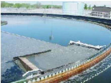
Waste Water Treatment Plant
